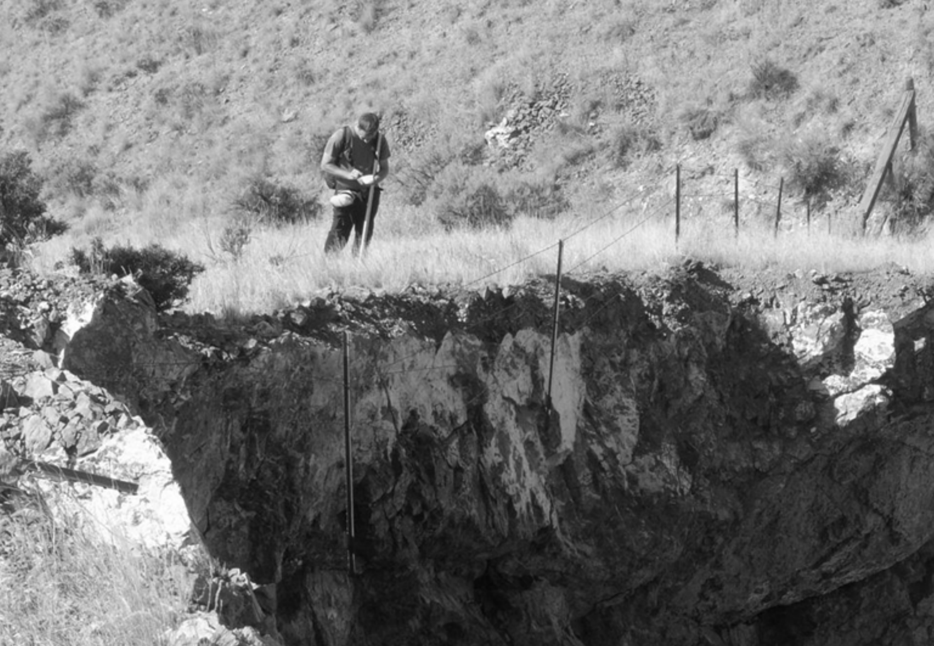
Figure 8. Fence has fallen into subsidence at MS118A (note the overhanging hazard).
